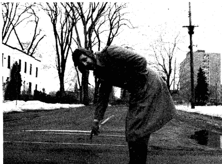
Will CITY HALL (in rear) disappear from the skyline? Sanitation department engineer J. T. Stools points to ominous cracks around personhole covers.
